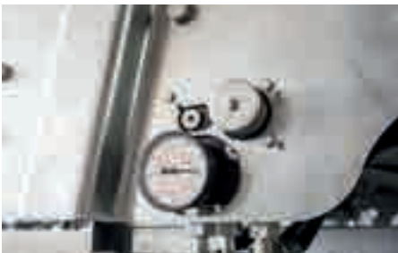
Mechanical feed control through mechanical potentiometer
