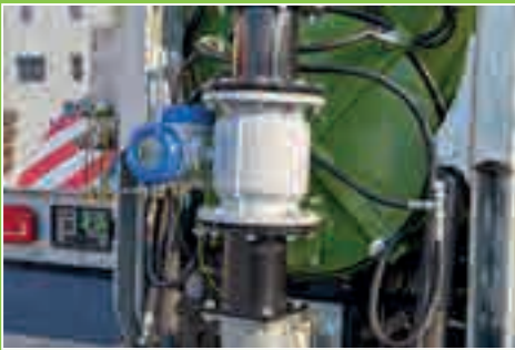
The flow rate during discharge is measured inductively by means of the Krohne Optiflux 2300 digital flow meter.
