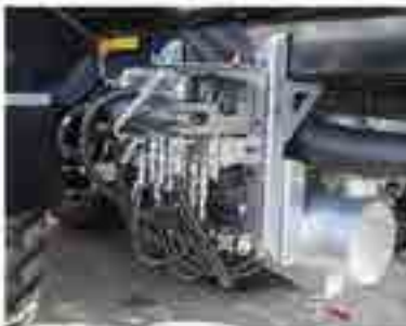
Hydraulic control block
